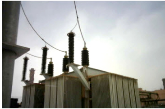
Figure 3 - Visual image of the transformer recorded with the IM500 daily snapshot.
